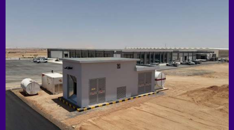
محطة خارجية بجوار المنشأة EXTERNAL SUBSTATION BESIDE THE FACILITY SOL is a trademark of Modern Distinguished Contracting Est.
