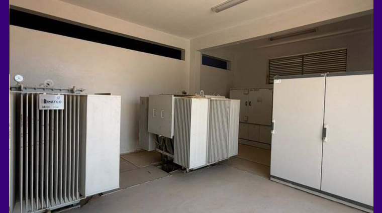
محول زيتي داخل غرفة الكهرباء OIL-FILLED TRANSFORMER IN THE ELECTRICAL ROOM SOL is a trademark of Modern Distinguished Contracting Est.
